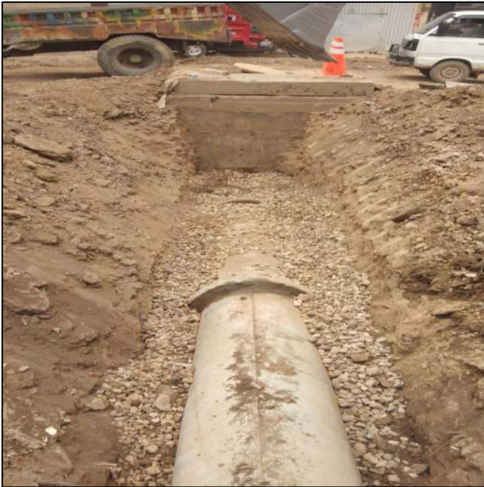
Picture 44: 18" i/d RCC Pipe Laying for Inlet Chamber Connection to Manhole @ Marala Road
