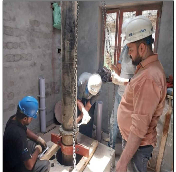
Picture 53: Lowering of Turbine & Motor Fixing of New Tube well P-27 Bonkan
