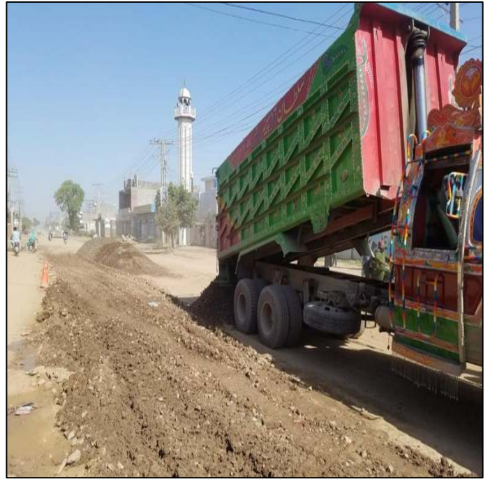
Picture 49: Restoration of Airport Road up to Sub Base Level is in Progress
