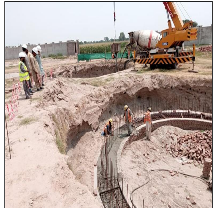
Picture 24: Supervision of Concrete pouring of screening chamber curb by EPCM and CIU
