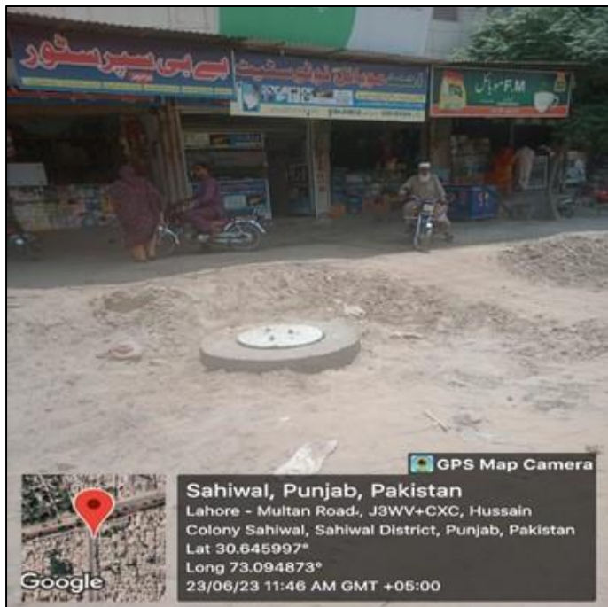
Picture 25: Installation of CI frame and Manhole cover at Line L-3.9.1 Arifwala Road
