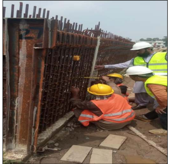
Picture 66: Checking steel dia, spacing of girder etc. before pouring of concrete
