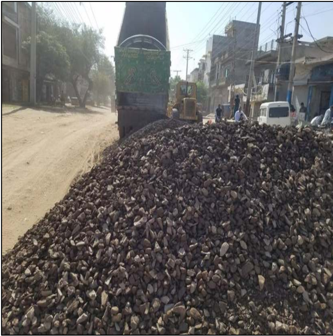
Picture 48: Restoration of Airport Road up to Sub Base Level is in Progress
