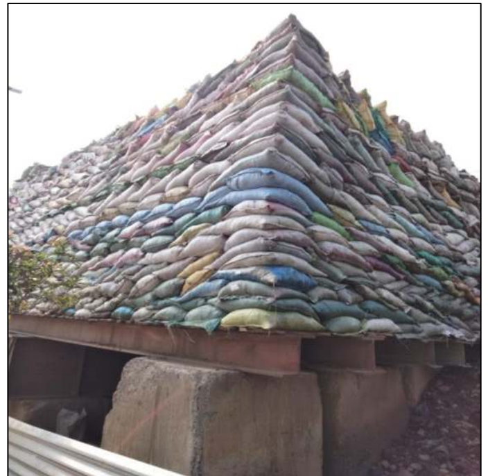
Picture 68: Platform Preparation for pile load test is in progress. 2x design load will be applied i.e., 800 tonne
