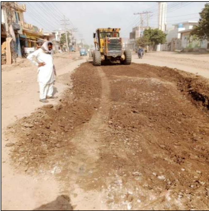
Picture 50: Gradation of Sub Base 2nd Layer is in Progress at Airport Road
